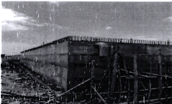
Figure 9: Mandera Water Supply Infrastructure- Reinforced Concrete Tank
