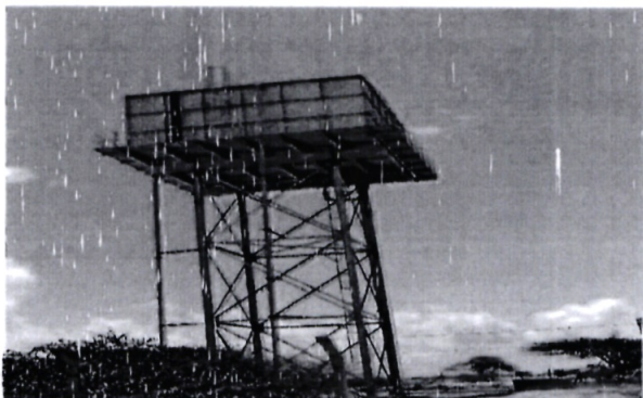
Figure 11: Garissa Water Supply Project-Iftin Girls Elevated Tank
