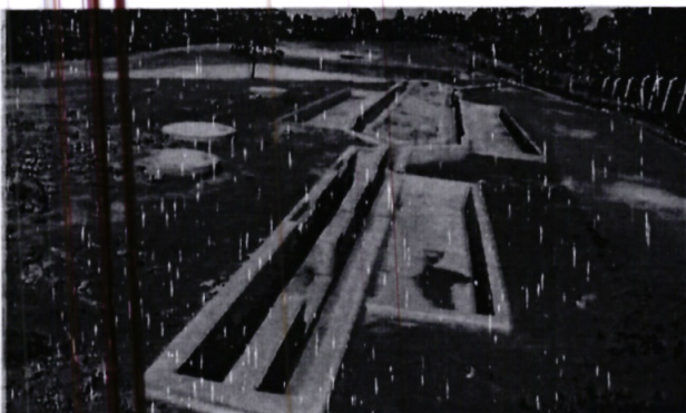
Figure 19: Chogoria Sewerage Infrastructure- Inlet Works
