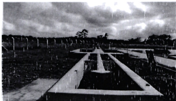
Figure 24: Kerugoya Kutus Sewerage Infrastructure - Inlet Works
