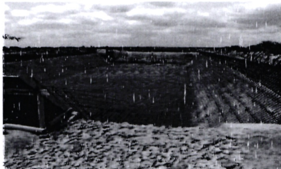
Figure 10: Mandera Water Supply Infrastructure Sedimentation Tank
