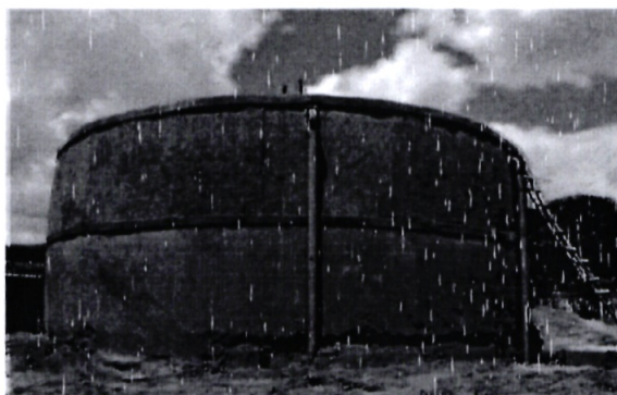
Figure 12: Garissa Water Supply Project- Storage Tank
