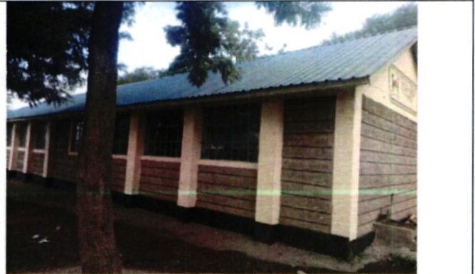
Eileen NgochochPri School - Renovation of 4 classrooms – Funded under emergency(Complete and in use)
