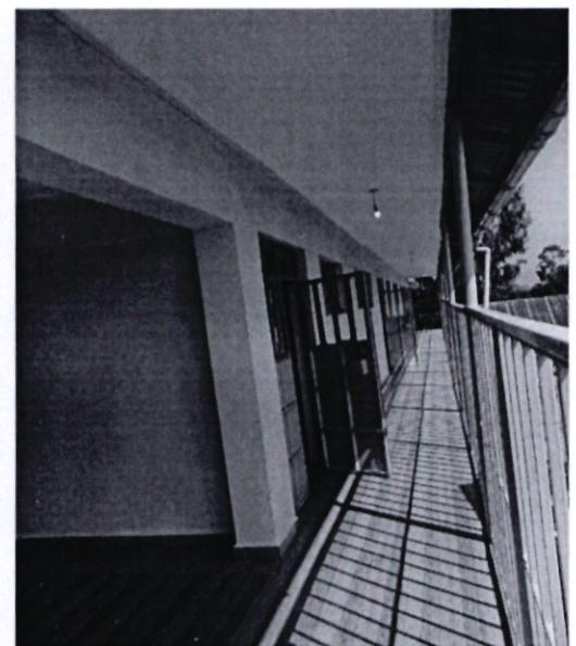
Construction of a story building made of 6No. Classrooms at Dunga Primary
