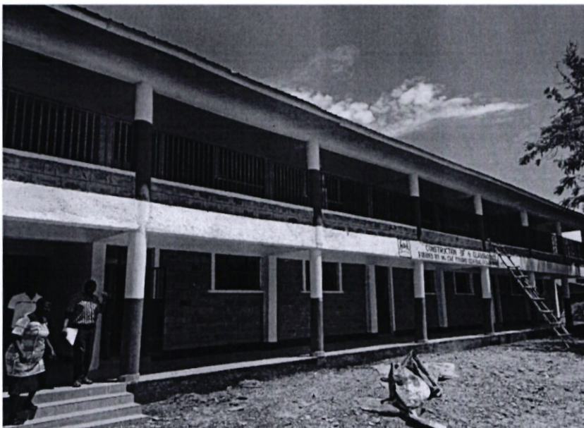
Construction of a story building Made of 6No. classrooms at PandPieri Primary School
