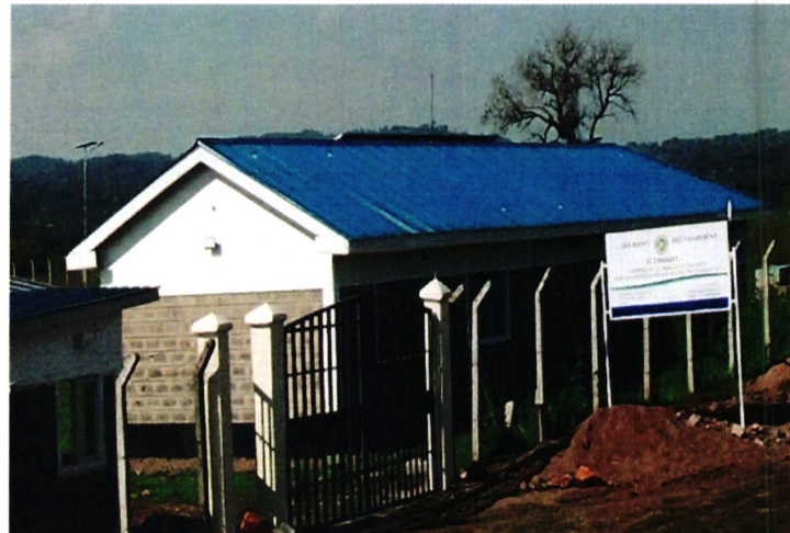
Chain-link fencing and farm house construction at Lichota Integrated Technology Transfer Centre
